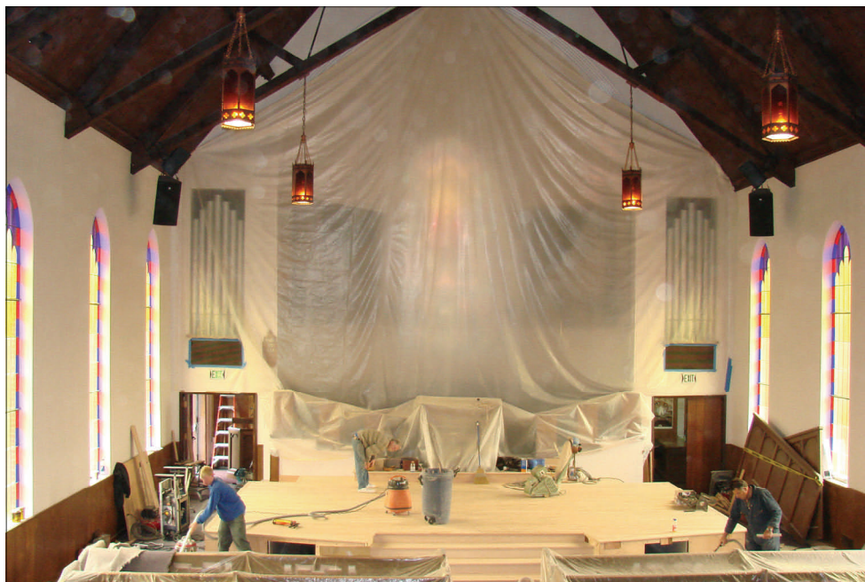
This photo, taken May 28, 2010, shows the platform enlargement in progress. The first service using the new platform will be June 5, when the orchestra plays for the first time without the old extenders. Photo by Carolyn Lacy
